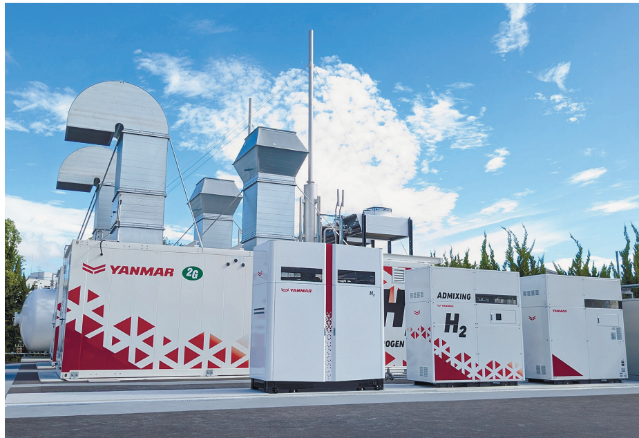
The Yanmar Clean Energy Site is a demonstration facility showcasing next-generation energy equipment.
