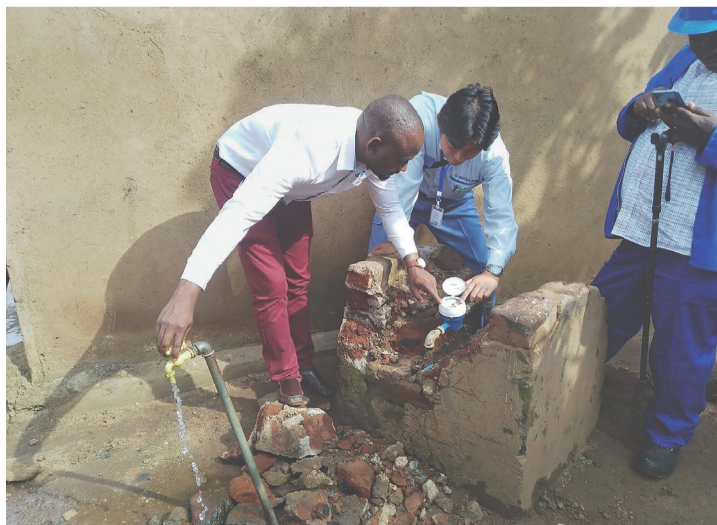
A Yokohama Waterworks Bureau employee shows a worker a new water meter in Malawi in 2019. YOKOHAMA MUNICIPAL GOVERNMENT
