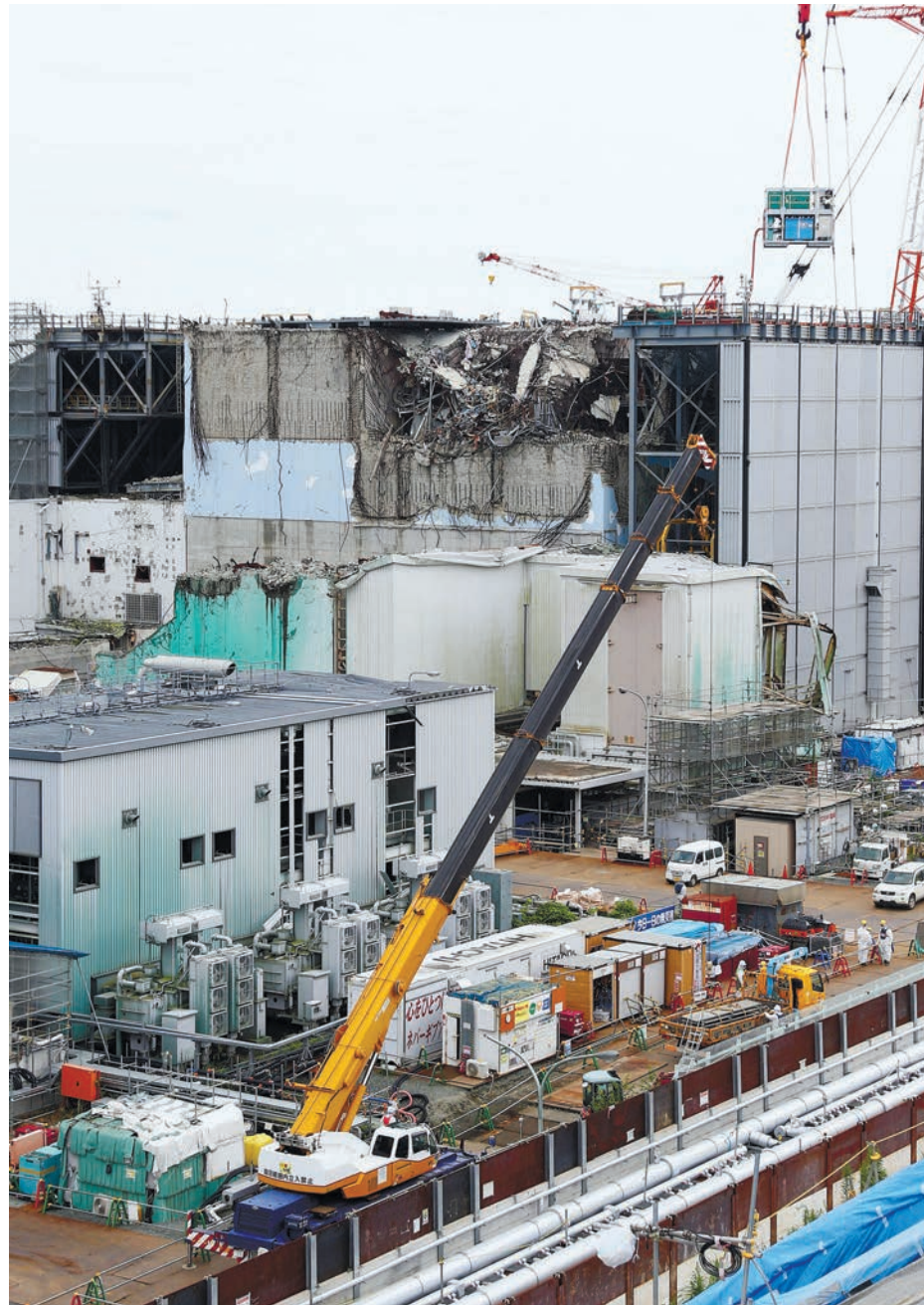
Tokyo Electric Power Co. crews work to clean debris at the Fukushima No. 1 power plant's No. 3 reactor on Sept. 4, 2015. KYODO
